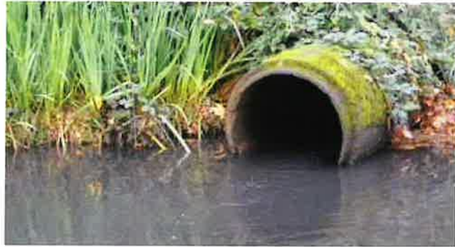
Factory drainage pipe in pond
